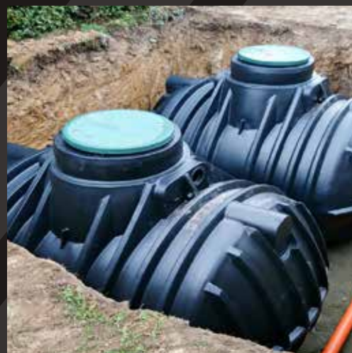
Septic Design & Installation
